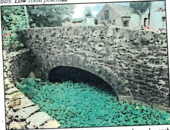
Plate 25 WC6 Stone Arch Bridge - Some cracks under arch offering limited opportunity. No evidence of bats. Low roost potential
