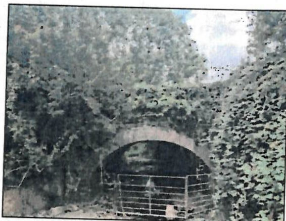
Plate 32 WC13 Stone Arch Bridge - Crevices and ivy cover noted. No evidence of bats. Low roost potential
