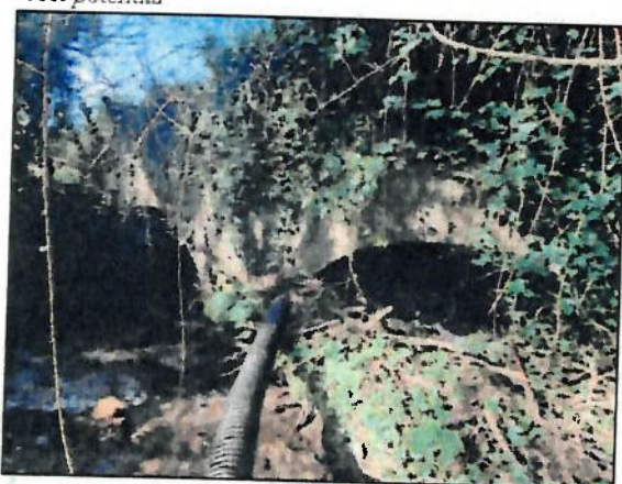
Plate 31 WC12 Stone Arch Bridge - Cracks and ivy present above/below bridge. No evidence of bats. Low roost potential
