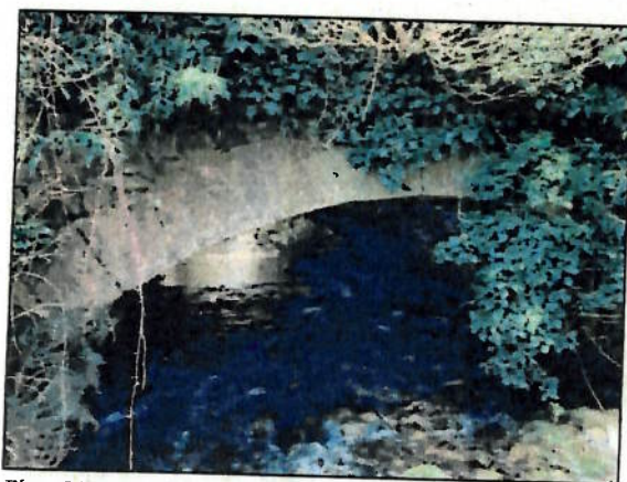
Plate 29 WC9 Stone Arch Bridge - Dense ivy on one side; cracks and crevices present. No evidence of bats. Low roost potential
