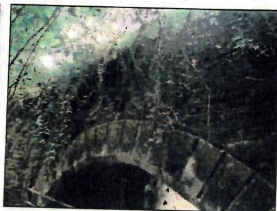
Plate 30 WC11 Stone Arch Bridge - Minimal cracks and ivy cover present. No evidence of bats. Low roost potential
